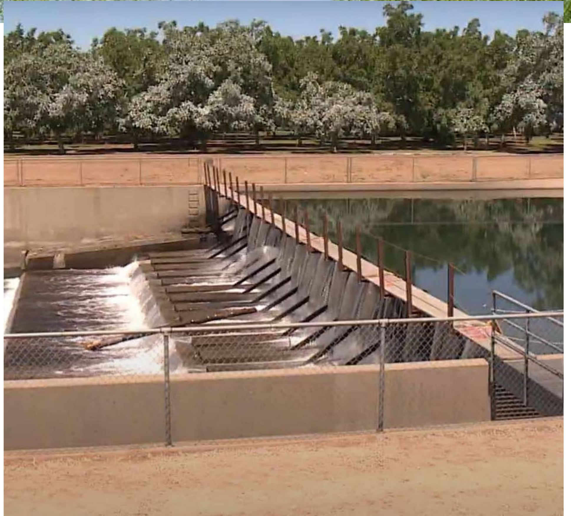
Gorrill Fish Screen and Ladder Project (credit: Gorrill Ranch)
